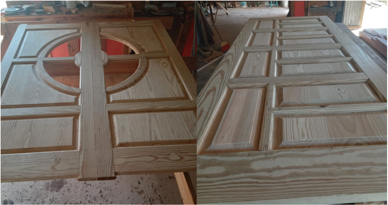
Close-up views of two doors that were being constructed for Codrington House.
