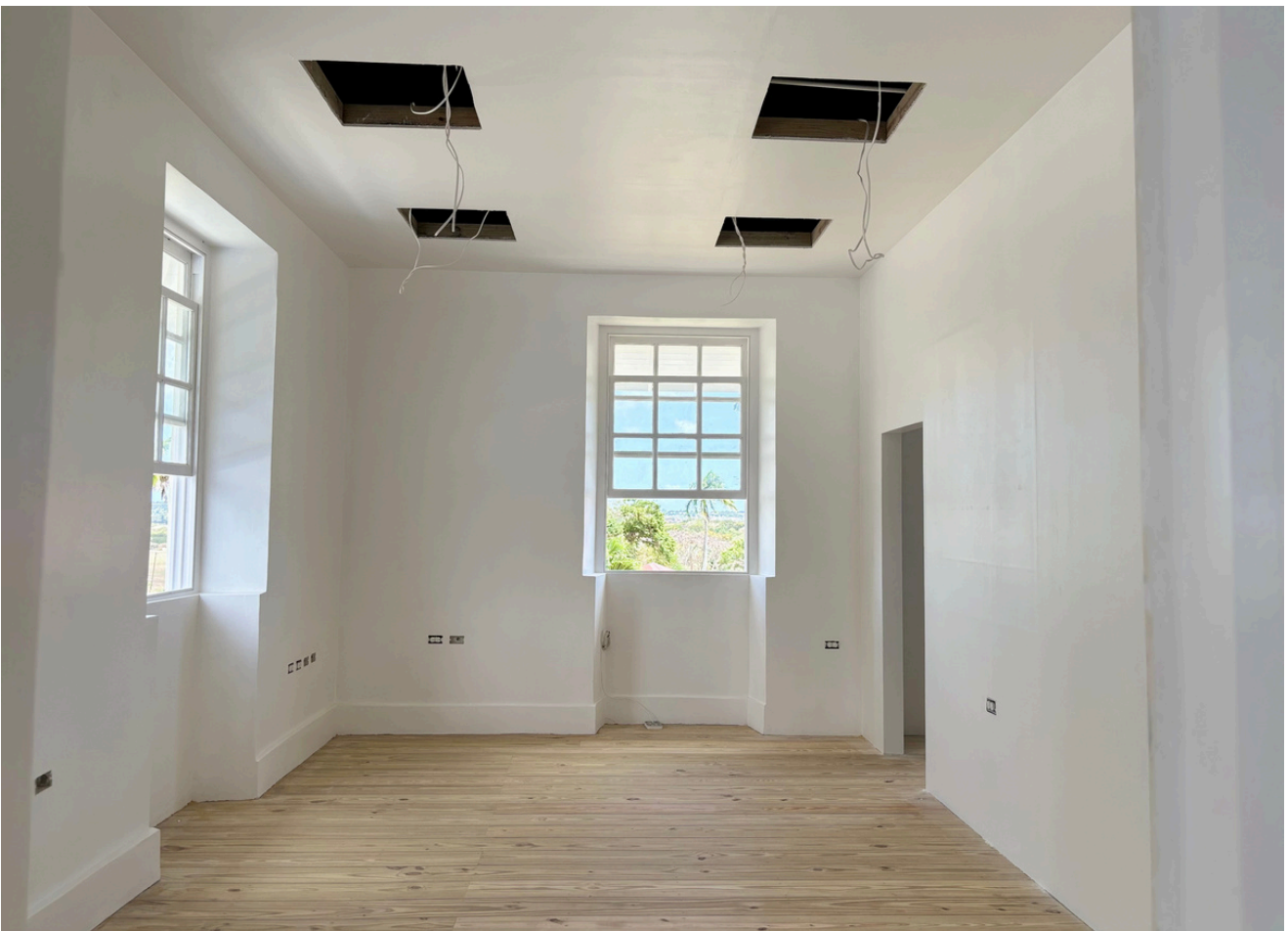
Another section of the Codrington House's interior wall after the repainting process.
