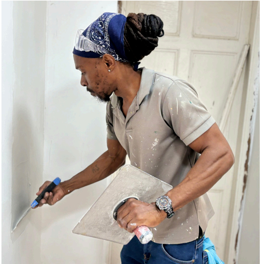
Patrick Hinds applying the slick compound to a wall in the Codrington House’s main office building.
