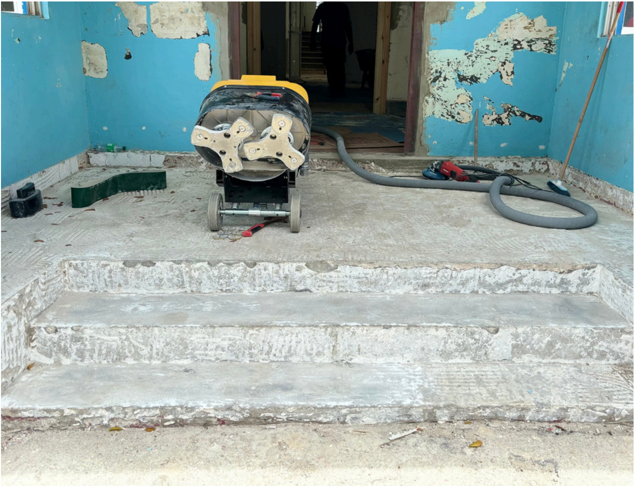
The Codrington House's entrance wall will also be repainted during this phase.
